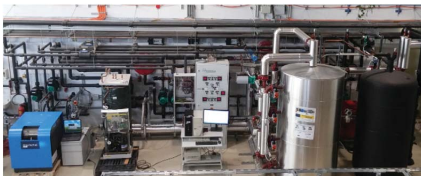
Heat pump test bench of the University of Applied Sciences Pinkafeld.
